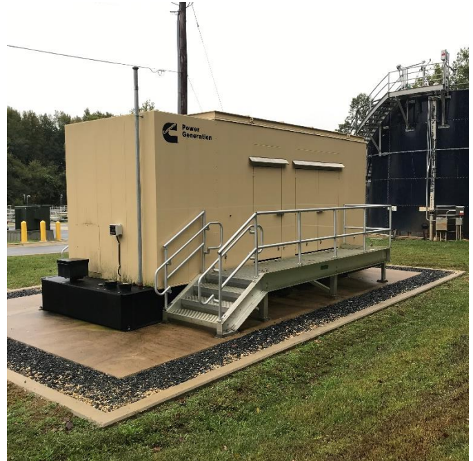
LEONARDTOWN WWTP GENERATOR
