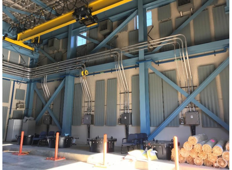
HUNTINGTON LEVEE PUMP ROOM RIGID ALUMINUM
