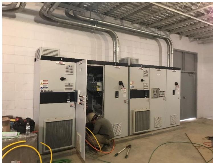
LITTLE HUNTING CREEK SPS VFD/RVSS
