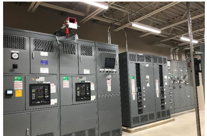
HUNTINGTON LEVEE ATS, SWITCHBOARD, & MCC
