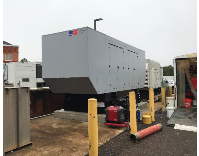
ST. MARY'S DETENTION CENTER GENERATOR
