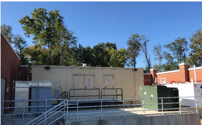
HUNTINGTON LEVEE GENERATOR
